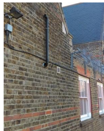
Flue height, shown in relation to ground floor windows at the rear of the northern school building (Mile End)
