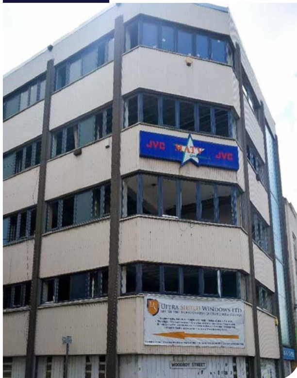
The appearance of MPK House on the site visit, with apparently stalled conversion
