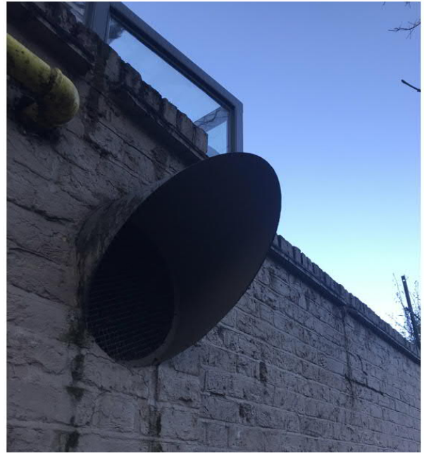
Kitchen ducts vent onto front playground.
