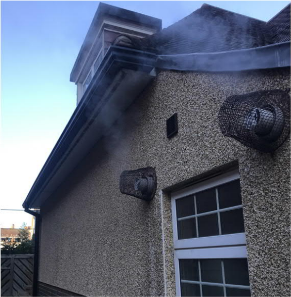
Boilers vent from the wall into the 2-year olds playground.
