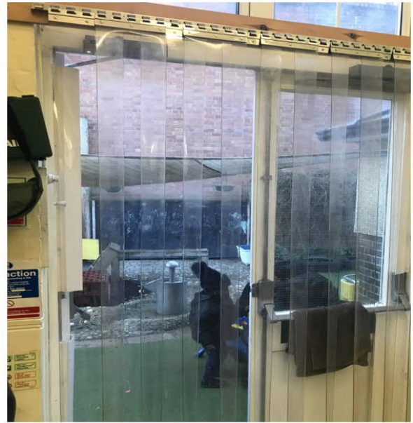
Doors opened throughout the day for free flow between classroom and playground. Butchers curtains are fitted to each doorway
