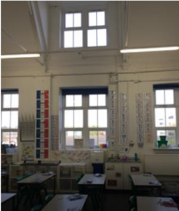
Large classrooms with poor insulation
