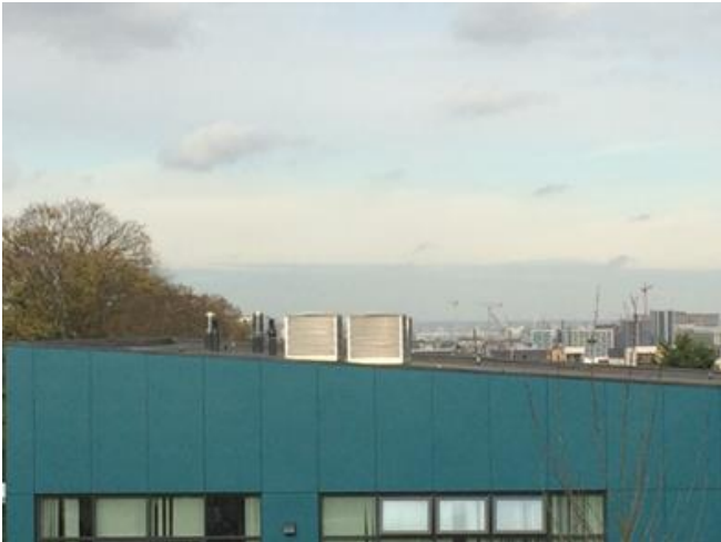
Air Handling Units and flues on the roof of the school hall building
