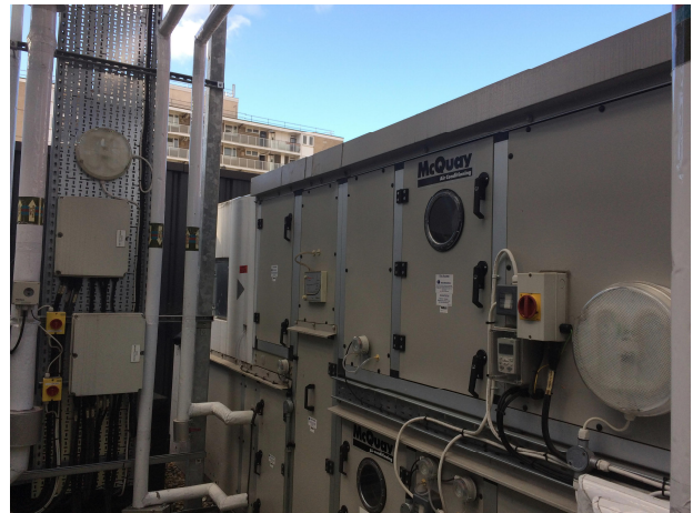
Air Handling Units on the roof of the new building
