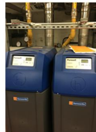
Boilers in main school building plant room
