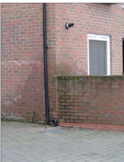
Some staining to brickwork on properties fronting Quilter Road.
