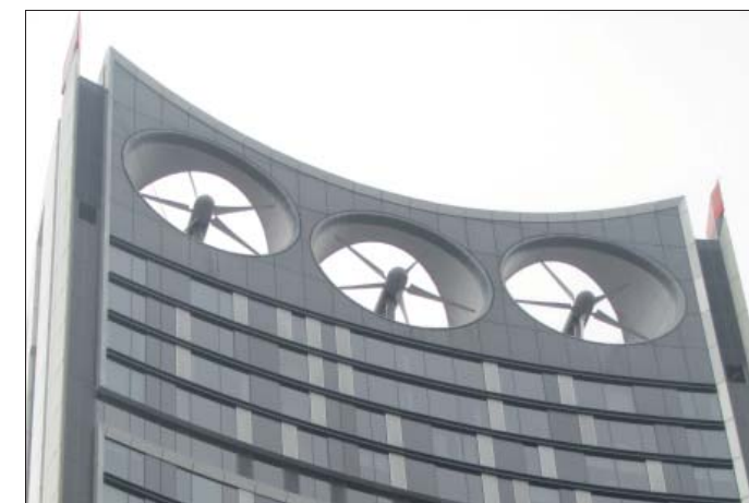
The wind turbines at the top of Castle House were not operational at the time of the visit.
